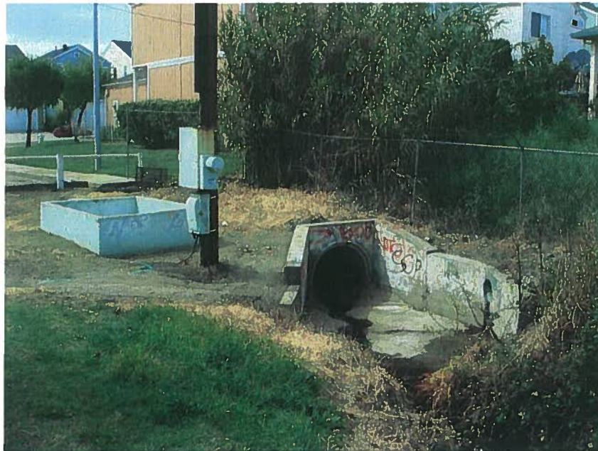
Figure 6-10 Hazel Street Pump Station
