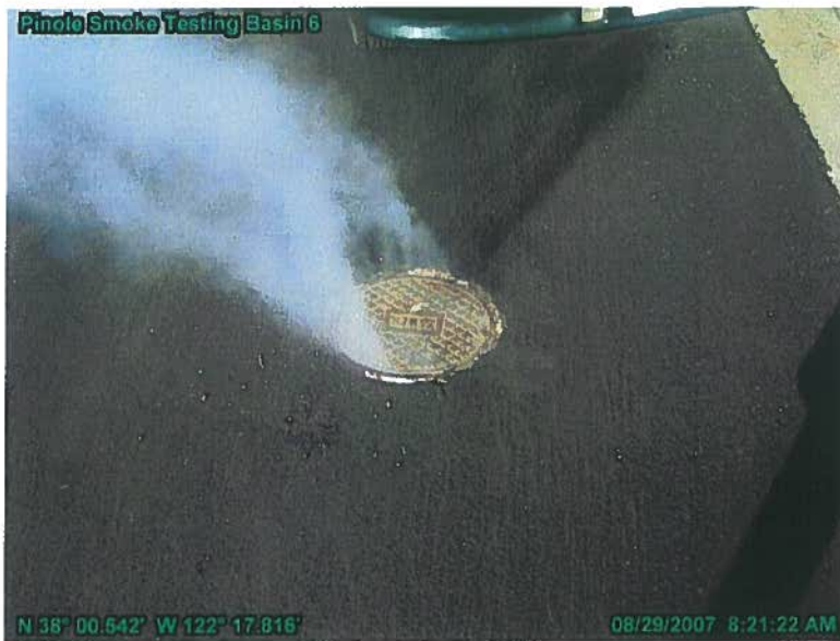
Figure ES - 4 Smoke Testing – Manhole If smoke can get out, then rain can get in.
